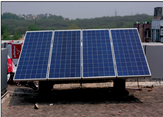
Roof top Solar Panel
